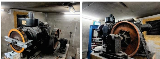
Fig. 5 Driving machine of passenger elevator
